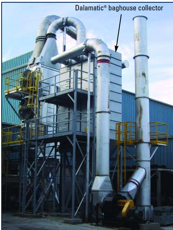
The Donaldson Torit Dalamatic® baghouse collector with GORE® REMEDIA® filter bags helps this recycler meet EPA regulations for dioxin and furan abatement.
