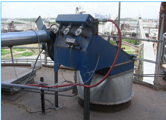
Torit PowerCore bin vents operate effectively on the grain holding silos at this barge unloading area.
